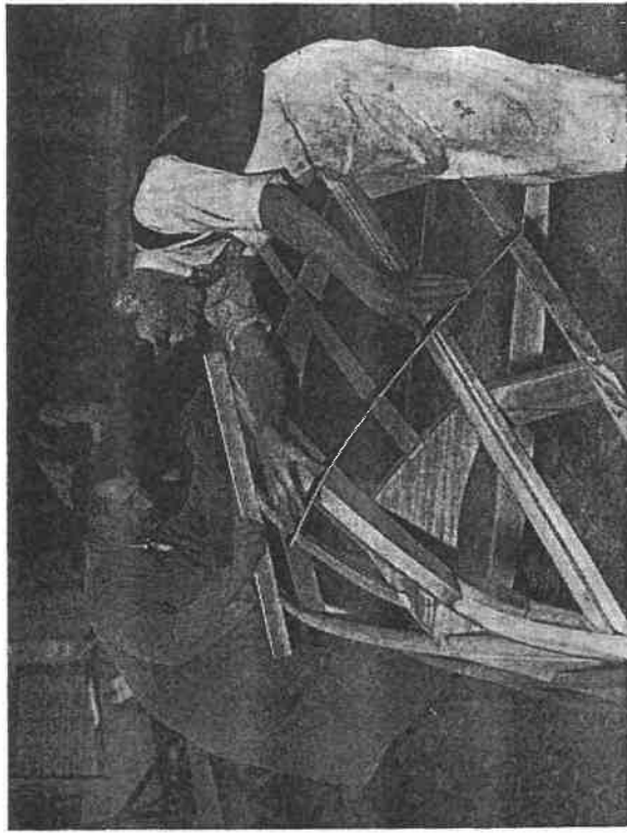
Fig. 6.—The process of fairing off straight and curved surfaces to receive the skin.
